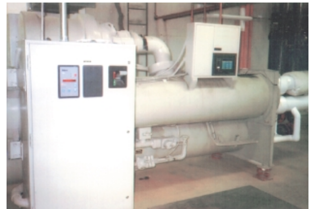
Figure 1 – Centrifugal Chiller and Controller
