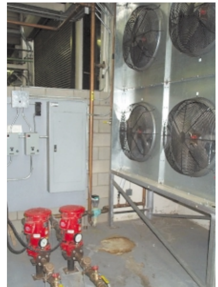
Figure 1 – Fan Coil, Pumps and Three-Way Valve
