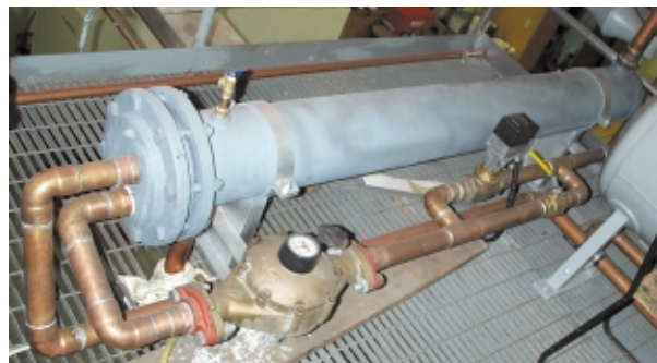
Figure 3 – Domestic Cold Water Heat Exchanger
