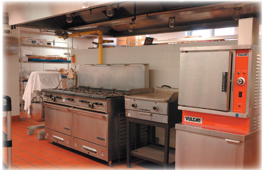
The Garland 280 Series gas range (above), Garland G22 Series gas griddle and Vulcan gas steamer all have a life expectancy of about twenty years. Buying energy efficient replacements will help save money and the environment. Effective January 2011, commercial ovens and griddles became eligible for the ENERGY STAR designation in Canada. As of the writing of this guide, the ENERGY STAR Simple Savings Calculator did not yet list ovens and griddles. For more details visit: www.energystar.gc.ca .
