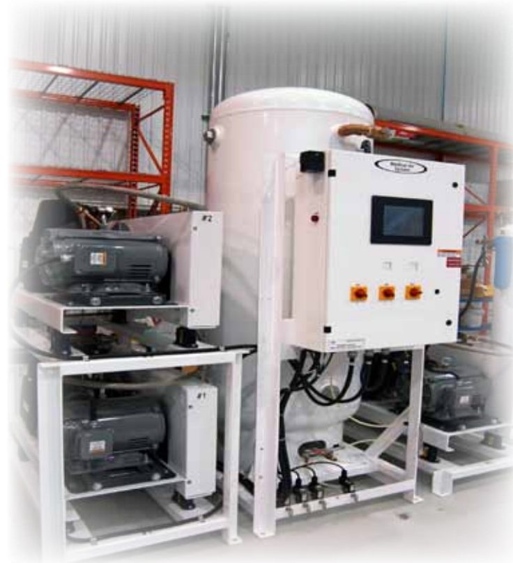
Class 1 Inc. medical air system in Toronto area hospital.
